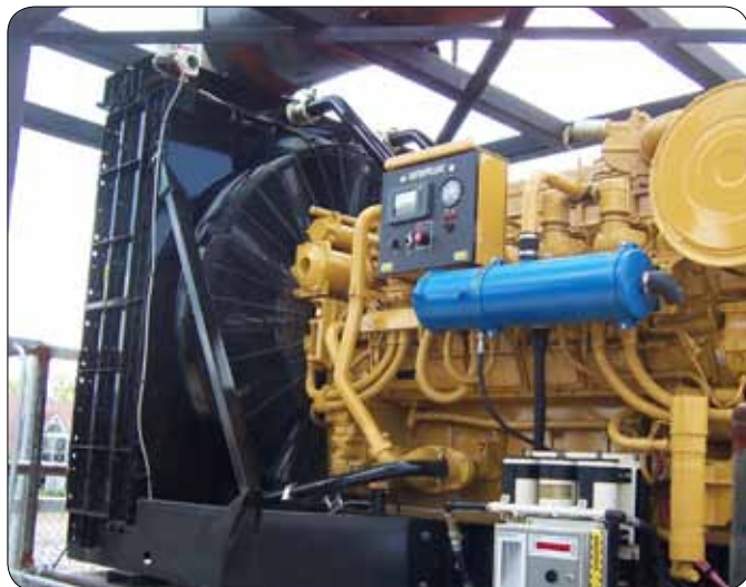
Pump Emergency Shutdown
