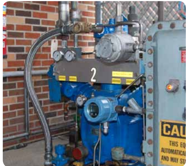
Gas Compressor Protection
